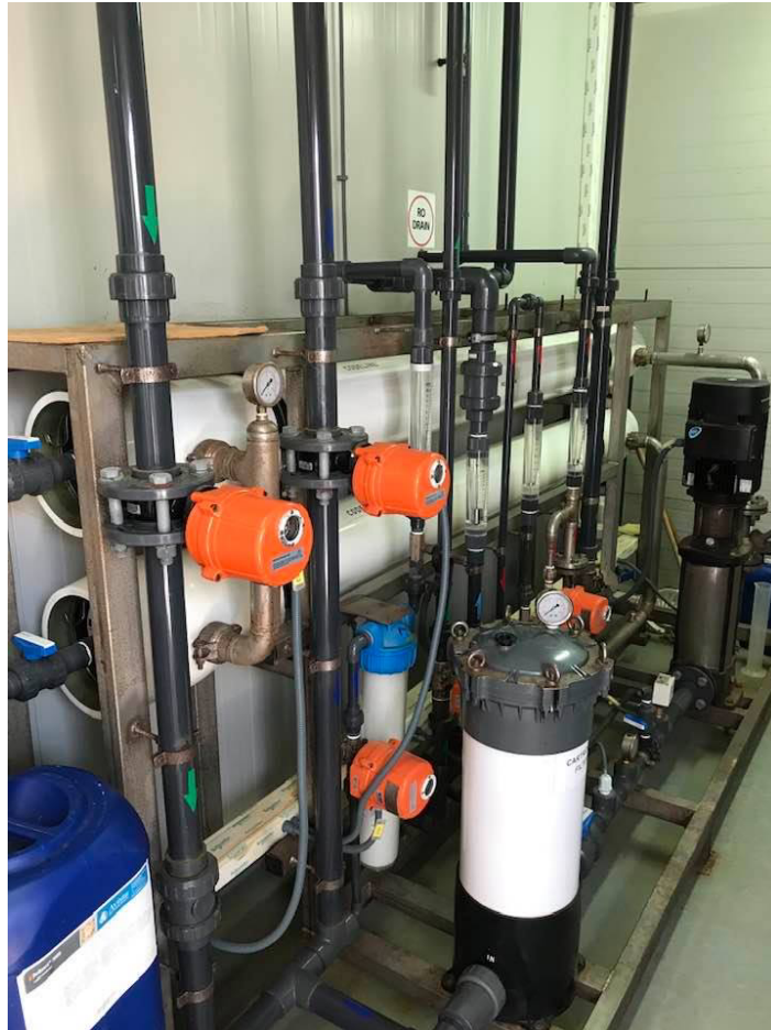
Reverse osmosis desalination unit at EJUST campus, providing safe and free drinking water
