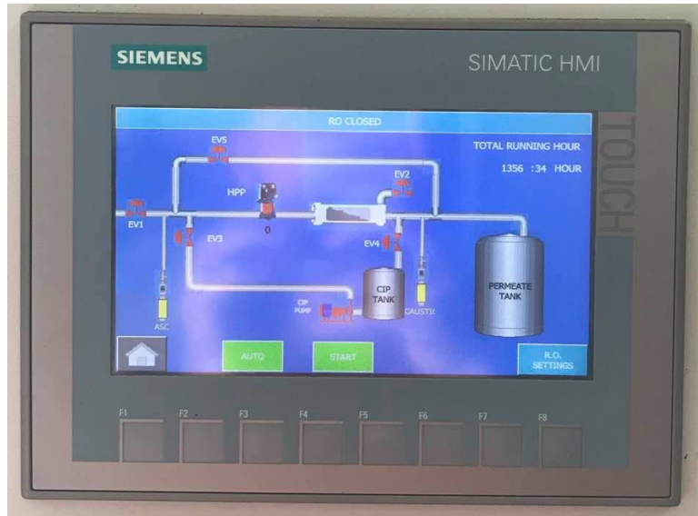
Automatic control and monitoring of the RO system
